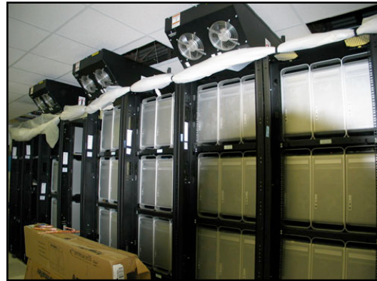
Fig. 7 - The cooling system used
